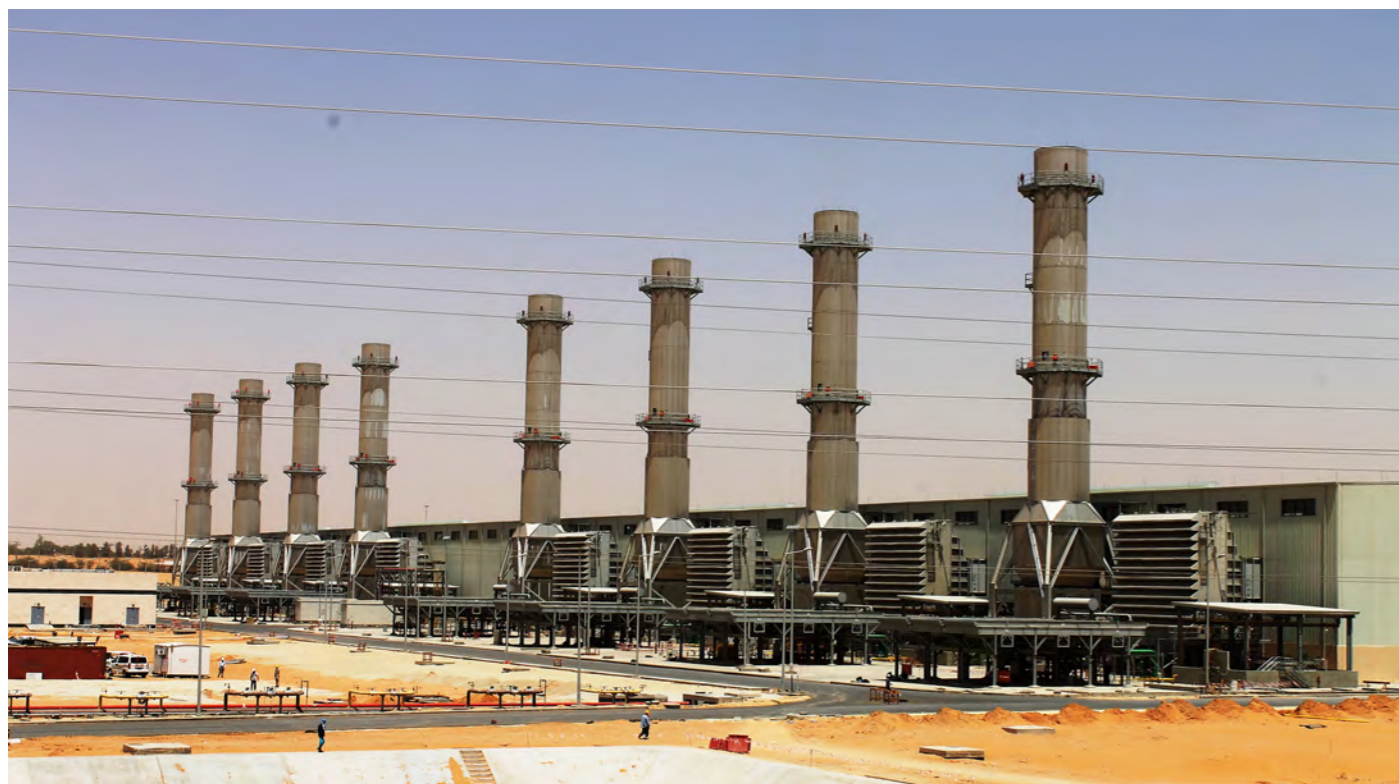
Qassim Power Plant Extension III
