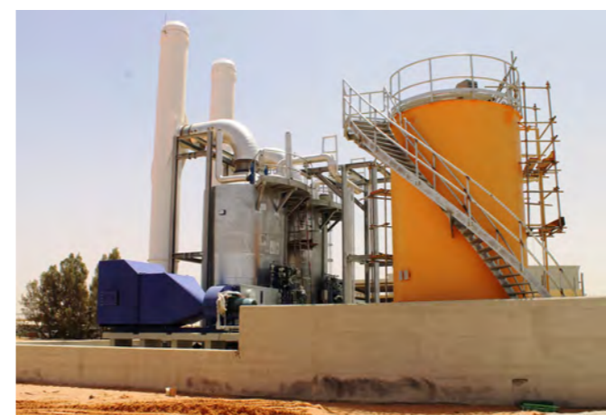
Boiler for Crude Oil Treatment Plant
