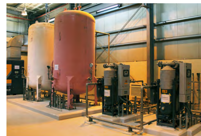
Compressed Air System
