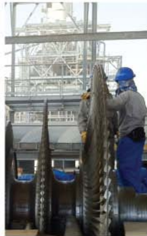
Steam Turbine, Qurayyah Power Plant
