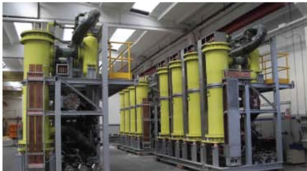
Electro-Chlorination Plant, Qurayyah
