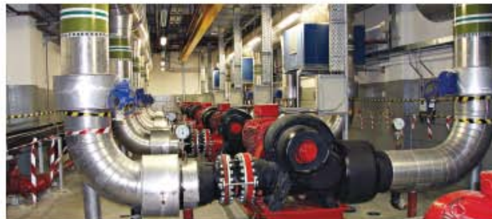
Qatar Cool West Bay, Doha
